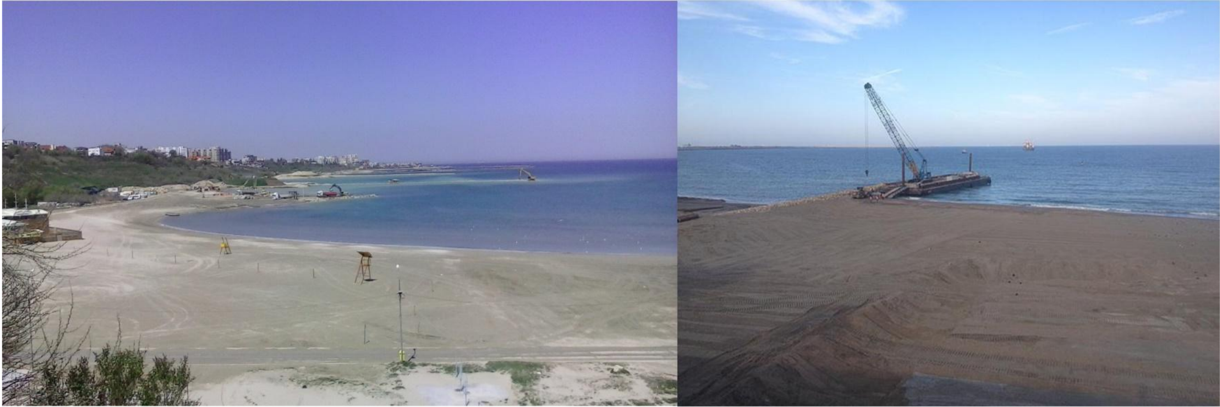
Beach protection and nourishment works in Tomis area (Constanta – April 2015) in the frame of the project `Protection and rehabilitation of the Southern Romanian Black Sea coast`
